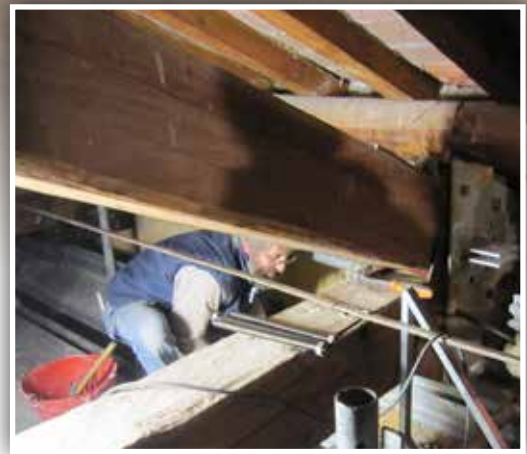
General view of the roof of the Refettorio during the implementation of the work
