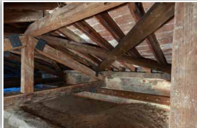
General image of the strengthening interventions on the roof over the corridor of the museum
