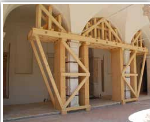
The provisional reinforcement of the columns of the main entrance of the museum in the "Secolari" cloister
