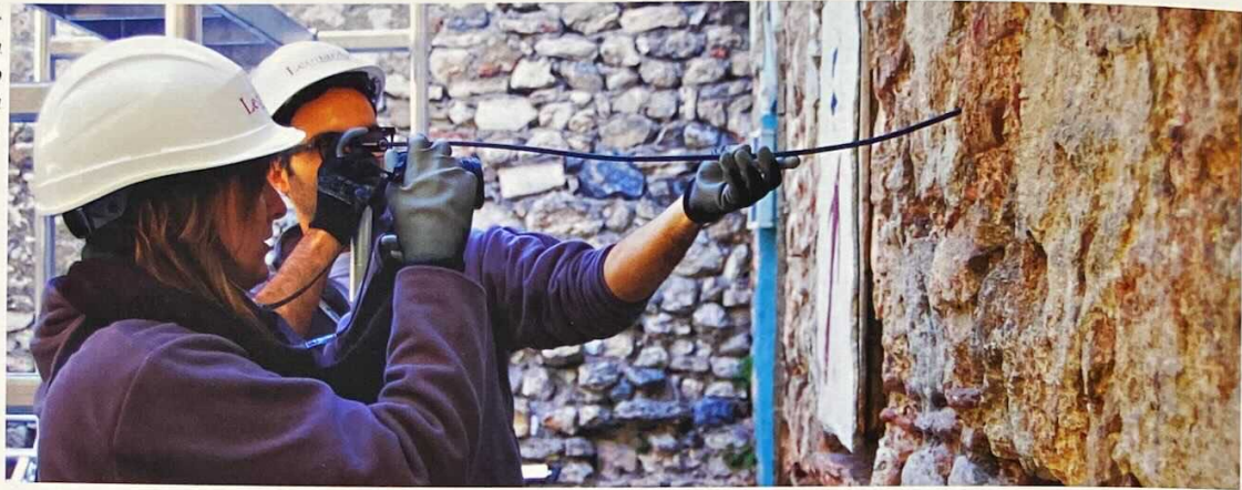
Figure 4. Examination of the micro cracks with camera.
